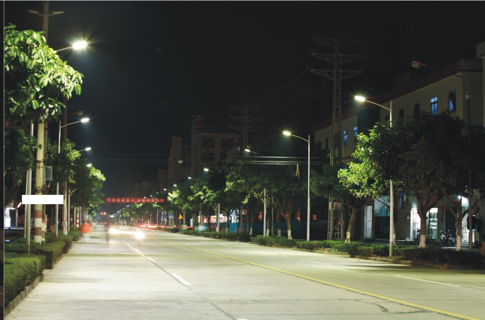
Street light project in Shilong town (4 lanes)
