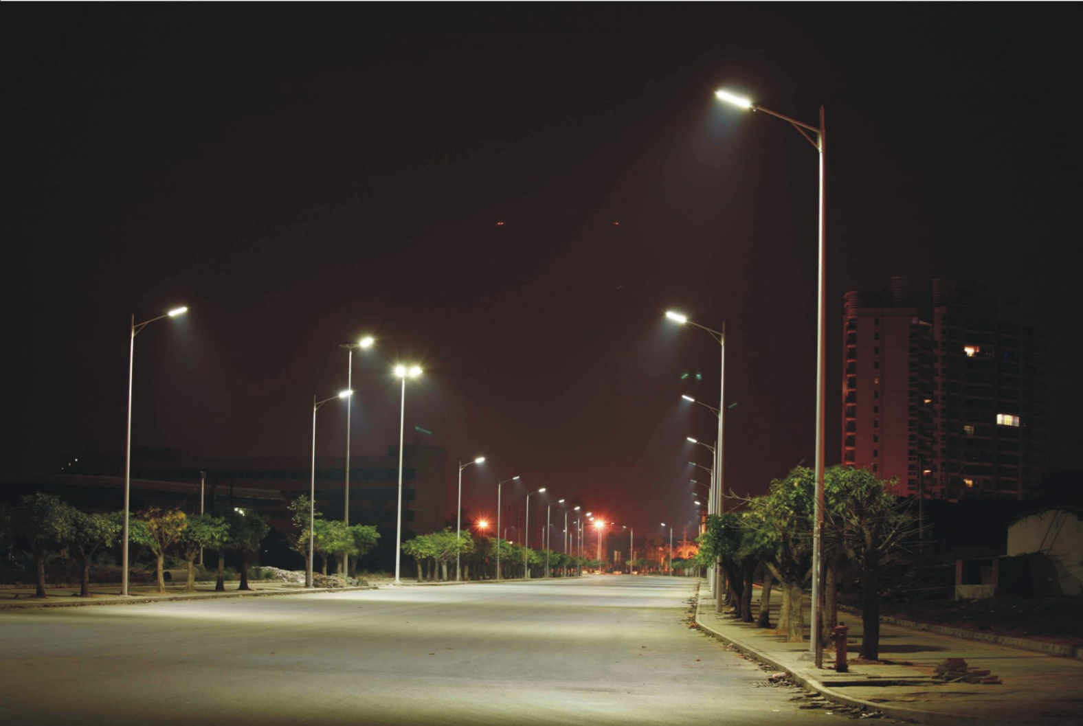
Street light project in Changping town (2 lanes)
