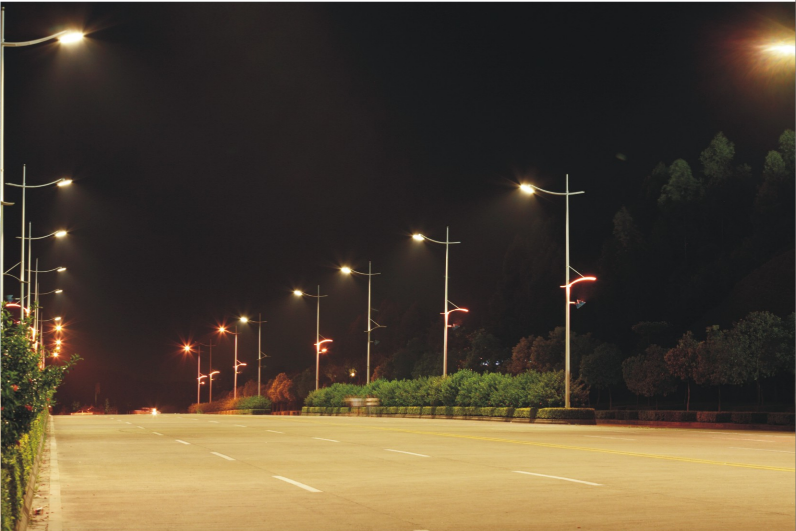
Street light project in Huizhou(6 lanes)
