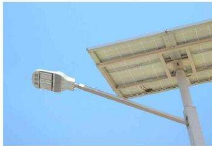
LED Street Light, LU2 in Mexico
