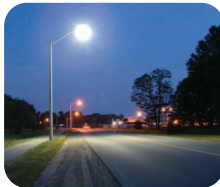
Remco's Bright LED Street Light is in the foreground and conventional HPS street lights in the background.
