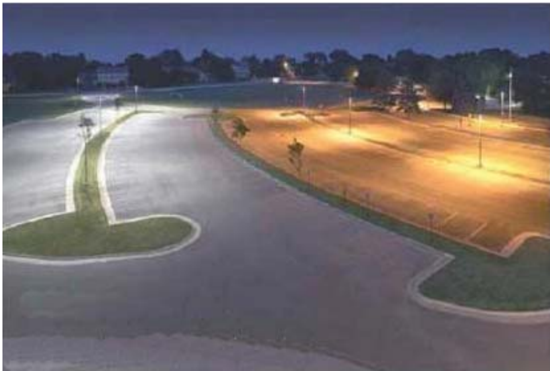
Left side of parking lot has 140 watt LED luminaires. Right side of parking lot has 300 W HID Luminaires.
