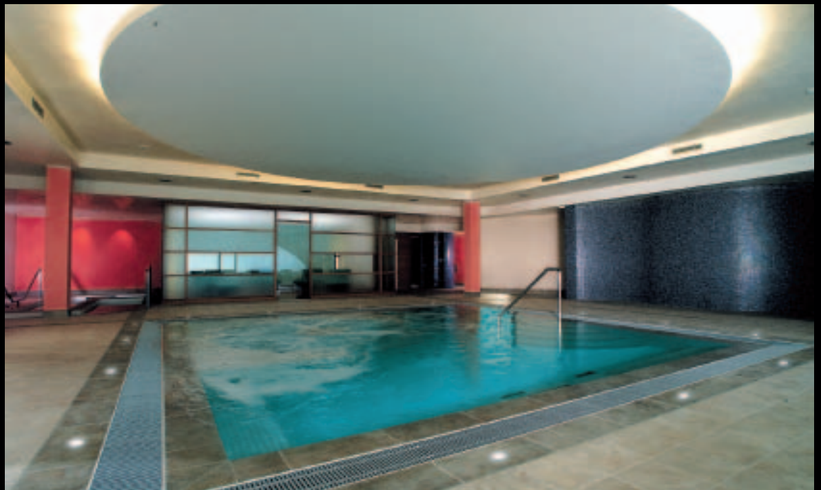
Private villa, lighting around the inside swimming pool IVELA built in lights
