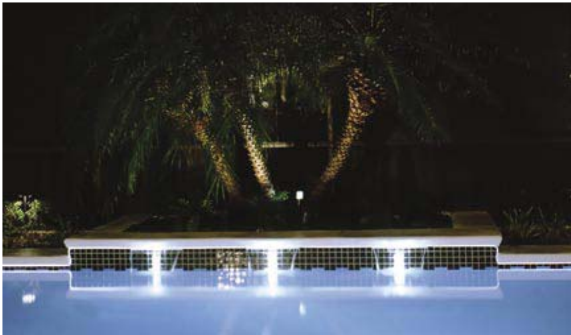
Feature light mounted behind sheet flow waterfall
