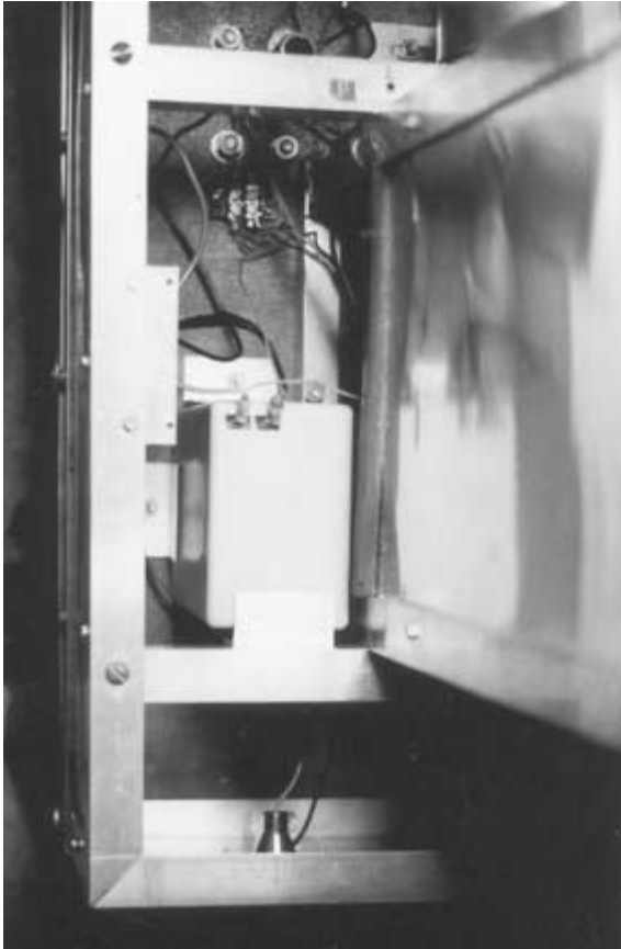
FIGURE 3-1. Location of one of the two 6-volt batteries.
