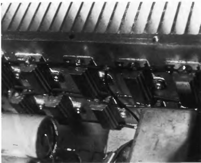
2.2 The author's resistor and heatsink combination. The resistors are finned and heatsink grease assists heat transfer to the heatsink.
